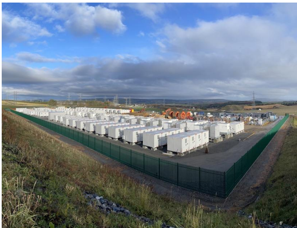
Figure 8.1: 349MW BESS located at Blackhillock, Scotland (Shutterstock: Rotorworx 1)
